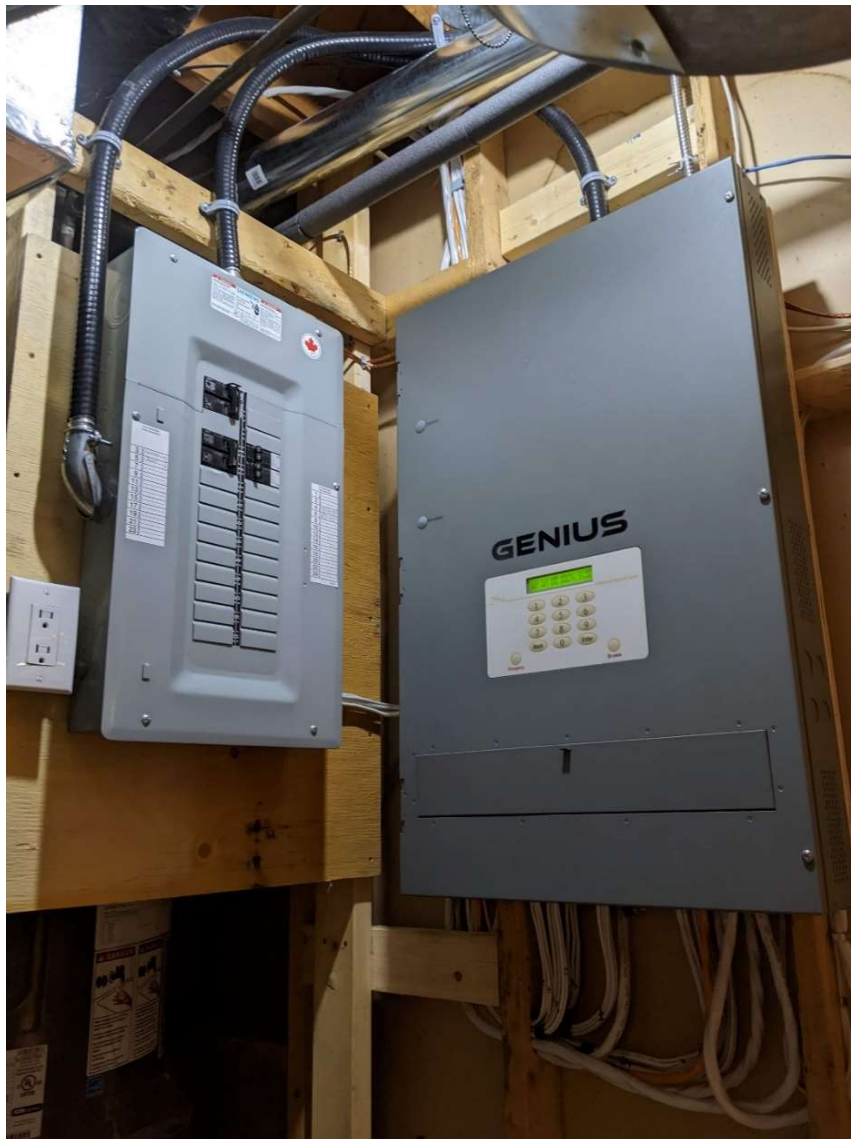
Photo: Koben Genius Smart panel installed as a sub panel
